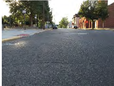
Water Street (Block 1) – Sidewalk is not flush with parallel handicap parking spaces.
