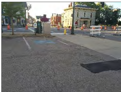
Troy Rec Lot (Non-ADA compliant) - A delineated aisle dedicated to the user does not exist.
