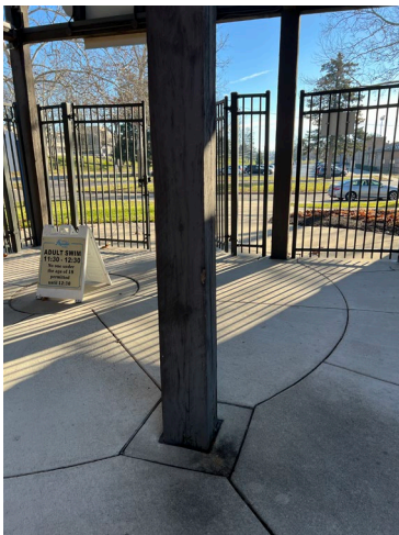
Wood Column Water Damage at Base
